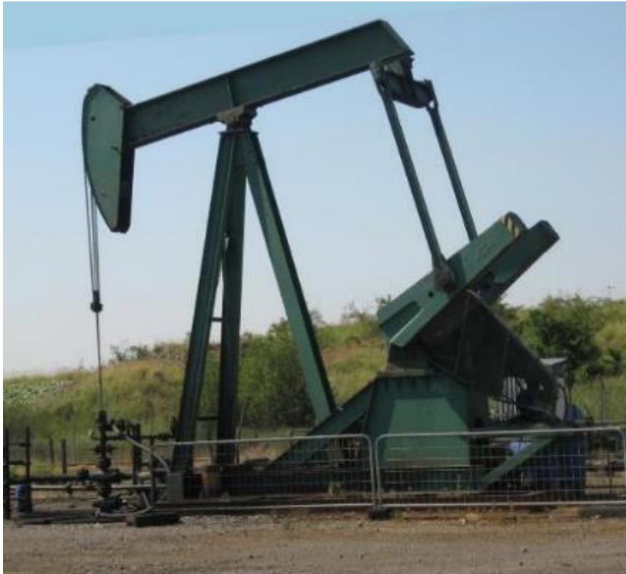
Photo shows a typical beam pump in operation at Europa's Crosby Warren site
